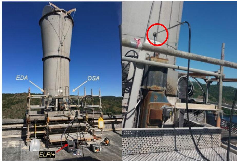
(a) (b) Figure 8 Test rig where (a) shows the stack with 3 sensors installed and (b) the detail of the probe for GS
