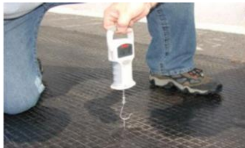
Figure 2.11 – Field test required in Australia for bond evaluation. Source: Department of Transport and Main Roads (2021).
