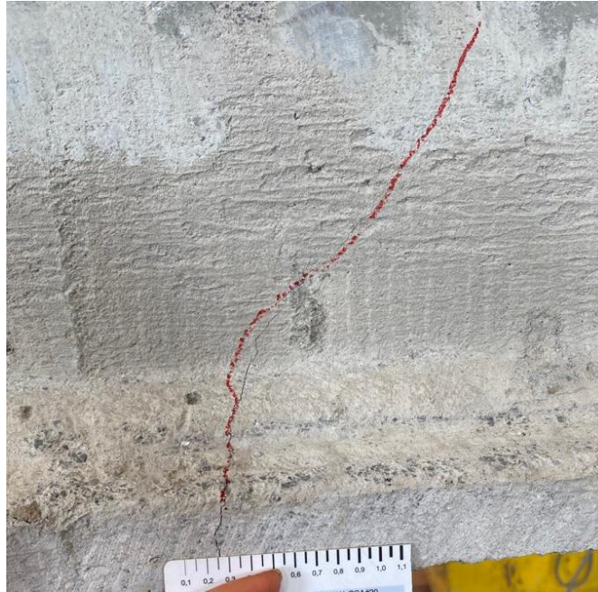
Figura 4.21: Fissura diagonal TA 05.
