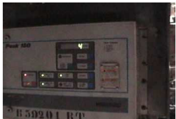
Painel Indicando Tripped e Front Panel
