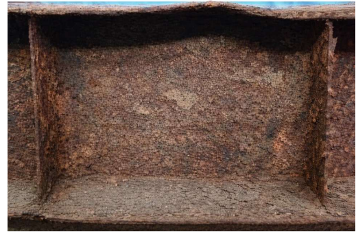
b) Failure mode of the beam with 10% corrosion (adapted from (Xiao et al. , 2023)).
