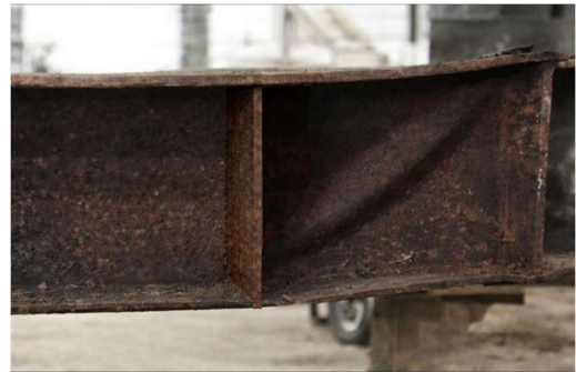
d) Failure mode of the beam with 12% corrosion (adapted from (Xiao et al. , 2023)).
